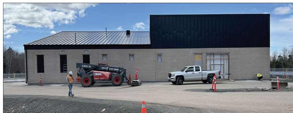
Springhill Wastewater Treatment plant. Photo by Acre Architects
