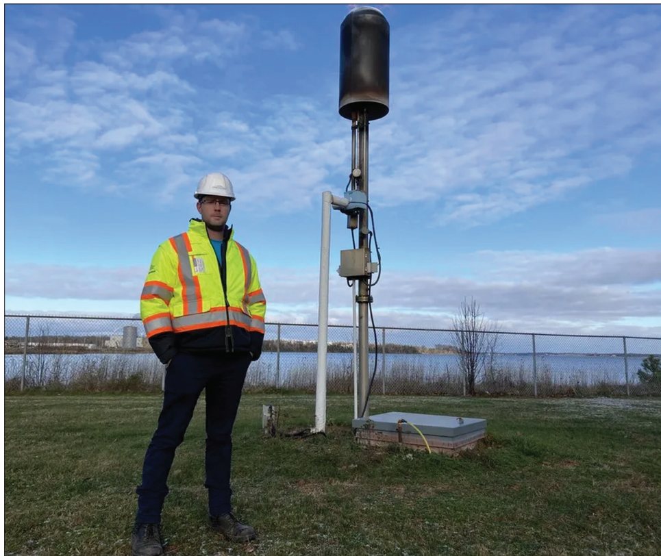
Charlottetown's water and sewer utility manager, Joshua McInnis, poses beside a flare at the city's Pollution Control Plant.
