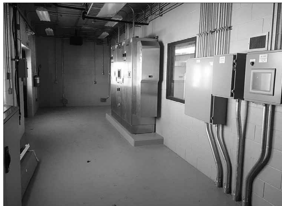
Inside the electrical control room of the UV building.
