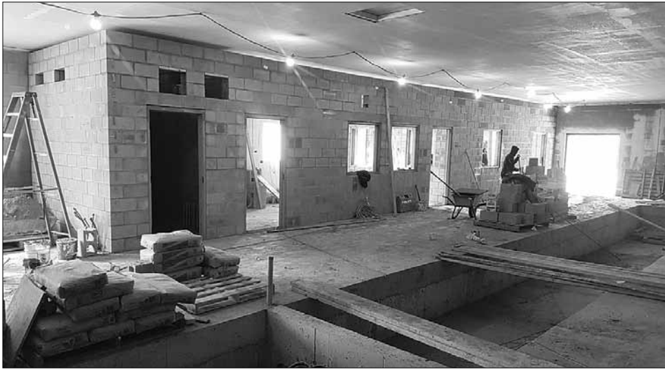
The new water treatment facility will include pressure zones to produce good water pressure throughout the town's higher and lower elevations.
