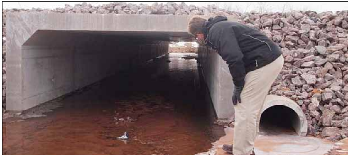
Aaron MacDonald, Summerside’s director of technical services, looks through a box culvert on South Drive.
