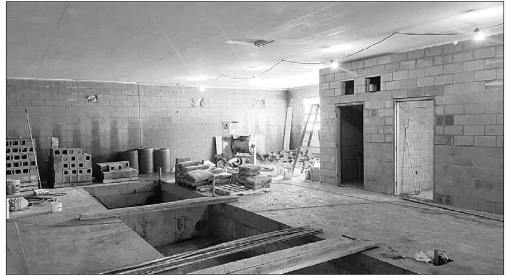
Pictou's new water treatment facility is expected to be finished by Sept. 1.
