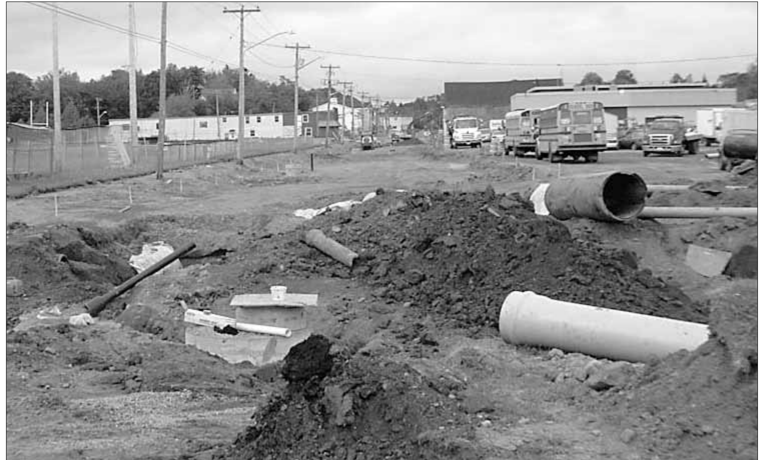
Sackville is currently working on its stormwater mitigation project, which will see the replacement of water, wastewater and stormwater mains in portions of the lowest elevation areas of the community. Here, crews work on a section of roadway, removing old iron pipes to install new PVC and concrete mains.
