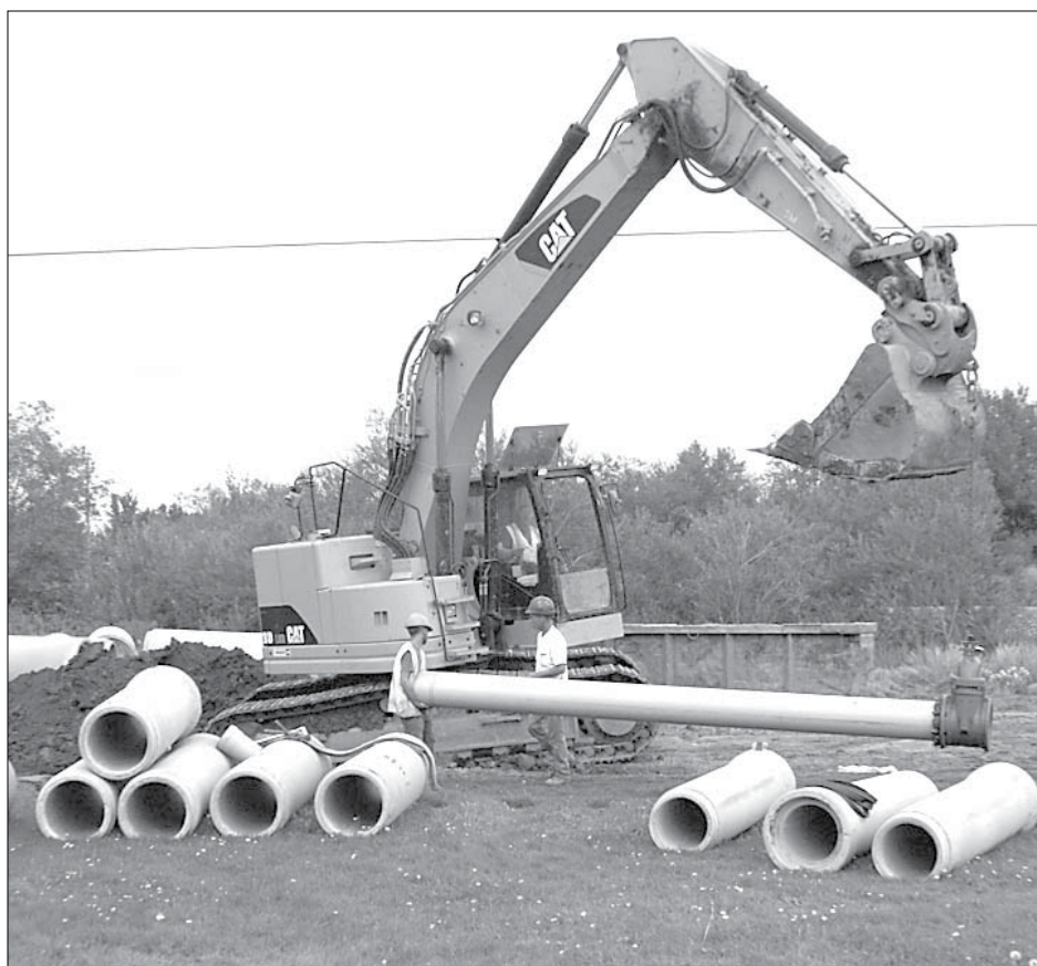
Bowser Construction Ltd. and Dexter Construction in partnership with Beal & Inch Construction Ltd. have been contracted to complete Phase One of that community's stormwater mitigation project. Shown here, owner Danny Bowser maneuvers the crane as his crew works to position a PVC water pipe into place on Lorne Street.
