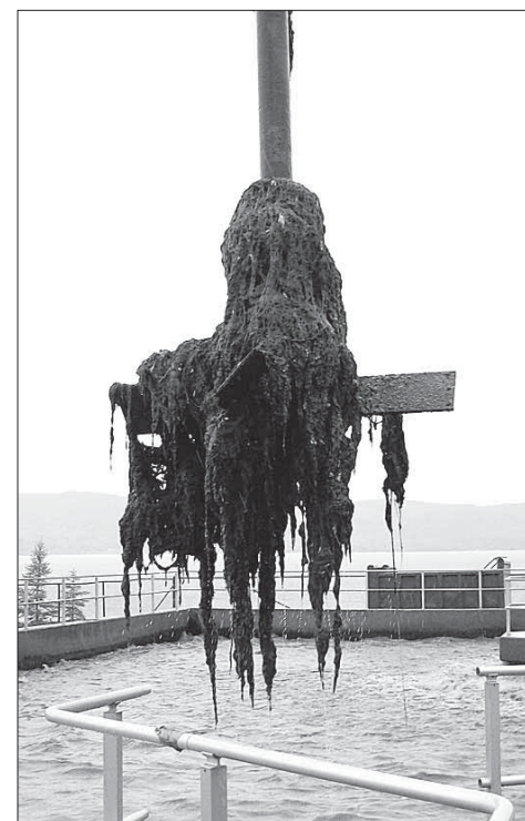
Before the new screen, the aerators (which look like large egg beaters) would become fouled with non-organic material tangled around the shaft, causing severe performance and maintenance issues.
