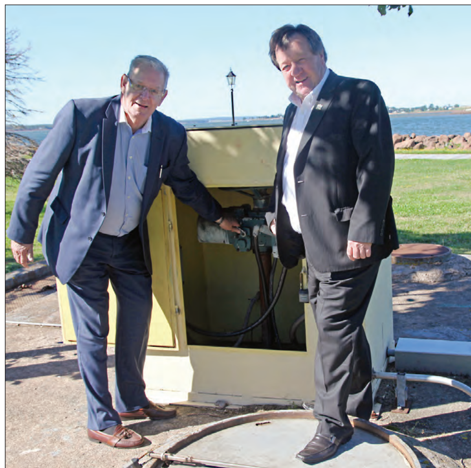
Councilor Edward Rice, chair of the city’s Water and Sewer Utility Department, and Charlottetown Mayor Clifford Lee turn off the Navy Quay regulator, completing the combined sewer separation project.
