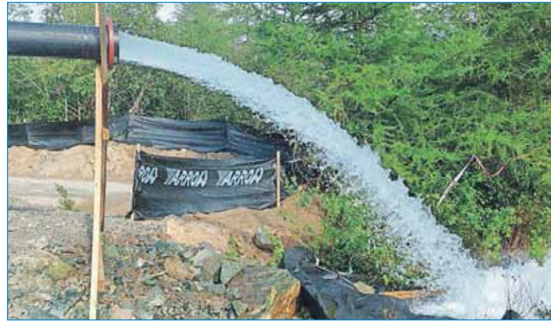
Water is flushed from one of three production wells that will supply the Saint John's West side with drinking water when the city's new water treatment plant is completed. - Submitted photo
