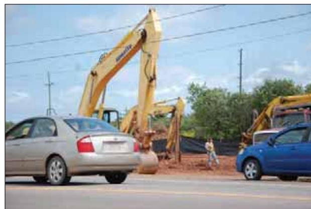
Crews work to install a new sewage pumping station at the North End of Granville Street in Summerside, Prince Edward Island. The new station is expected to be completed by early November and will increase capacity for that part of the city. (Photo: Colin MacLean/Journal Pioneer)
