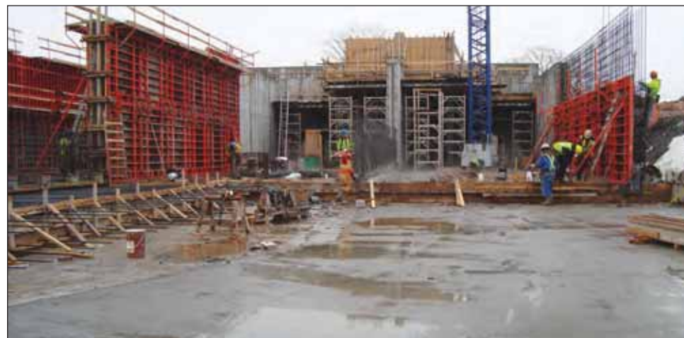
The design/build project contractor for the Eastern Passage Wastewater Treatment Facility was Maple Reinders Constructors Ltd. of Mississauga Ontario and Maxim 2000 Construction Inc. based in Dartmouth, Nova Scotia. (Photo: Maple Reinders Maxim Joint Venture)
