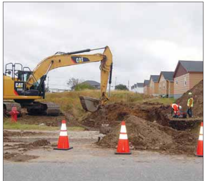
An excavator operator with Boyd & Bungay Construction Ltd. digs near Prince Rupert Drive in Stephenville, Newfoundland & Labrador Sept. 24 for the laying of storm sewer pipe. Another employee works at starting a generator to provide power for tools used in laying the pipes. It's all part of the first phase of Grove Street Reconstruction. (Photo: Frank Gale/Western Star)
