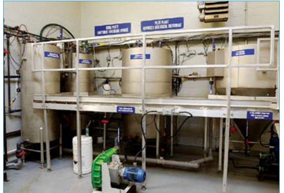
The Greater Moncton Wastewater Commission's 'Pilot Plant'. (Photo: Contributed)
