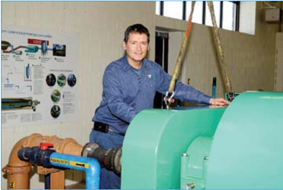
Burtis Hayes works on a centrifuge in the Dewatering Building at the Greater Moncton Wastewater Commission. (Photo: Contributed)
