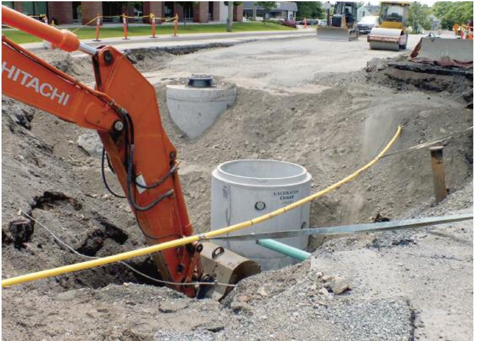
A storm sewer was installed on Somerset Street and Wellesley Avenue in Saint John, New Brunswick this summer. (Photo: Carmel Vivier)
