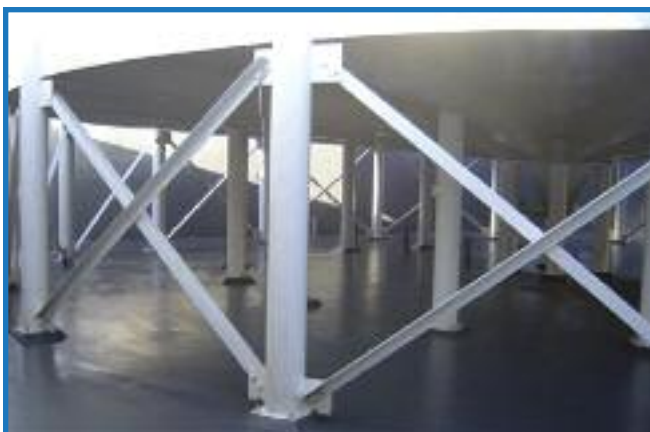
The ongoing integrity of many water and wastewater containment structures depends on the abilities of the containment system linings—such as the Elasti-Liner system from KCC—to provide protection against leakage over time. The photo shows a containment area for sulfuric acid.
