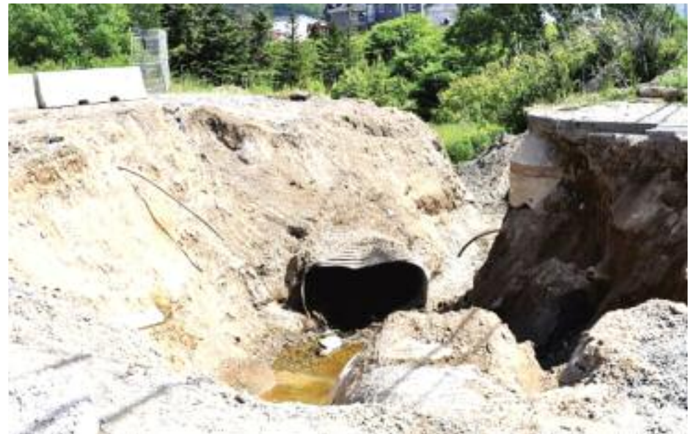
City of Corner Brook staff was busy in July when a sinkhole between 10 and 12 feet deep appeared on Country Road. They discovered that the storm pipe running under the road had deteriorated and that a waterline in the area was leaking. (Photo: Diane Crocker/Western Star)
