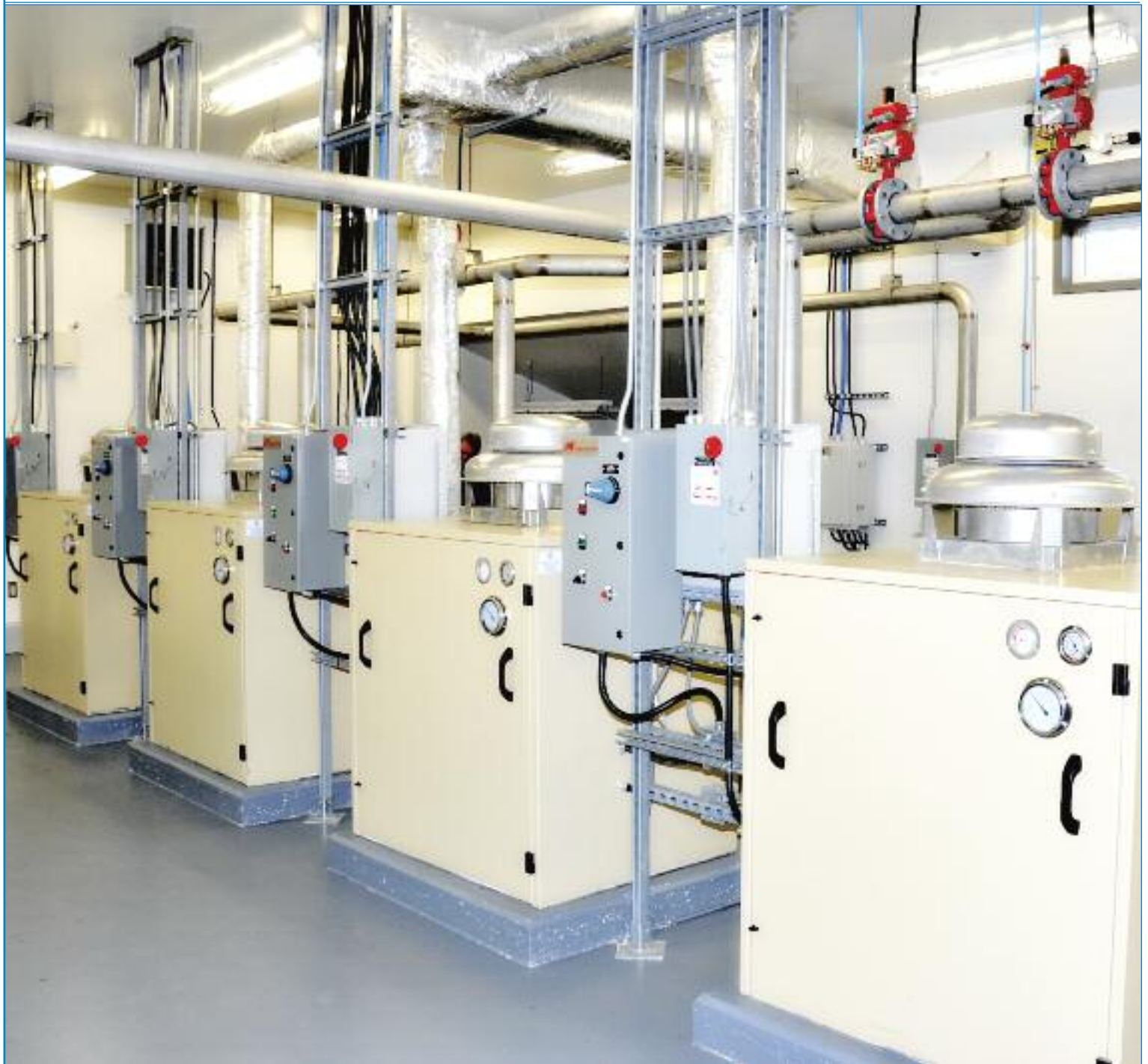
The Havre Boucher Wastewater Treatment Facility officially opened in December. (See the story on page 3) (Photo: Contributed)
