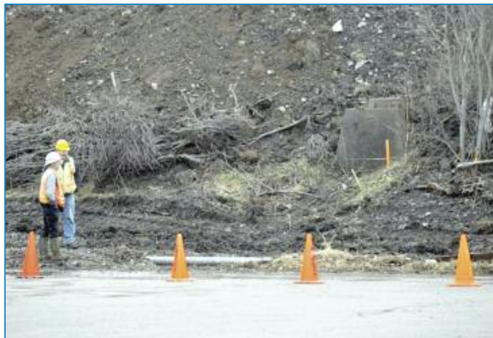
On Dec. 11 Caldwell and Ross Limited employees survey the area surrounding Exit 24 where the company is working to replace a damaged culvert and repair the walking trail behind Sobeys head office in Stellarton, Nova Scotia. The company was awarded a $4.3 million contract from the province to complete the work and is expected to finish the job by June 30. (Photo: Amy MacKenzie/The News)
