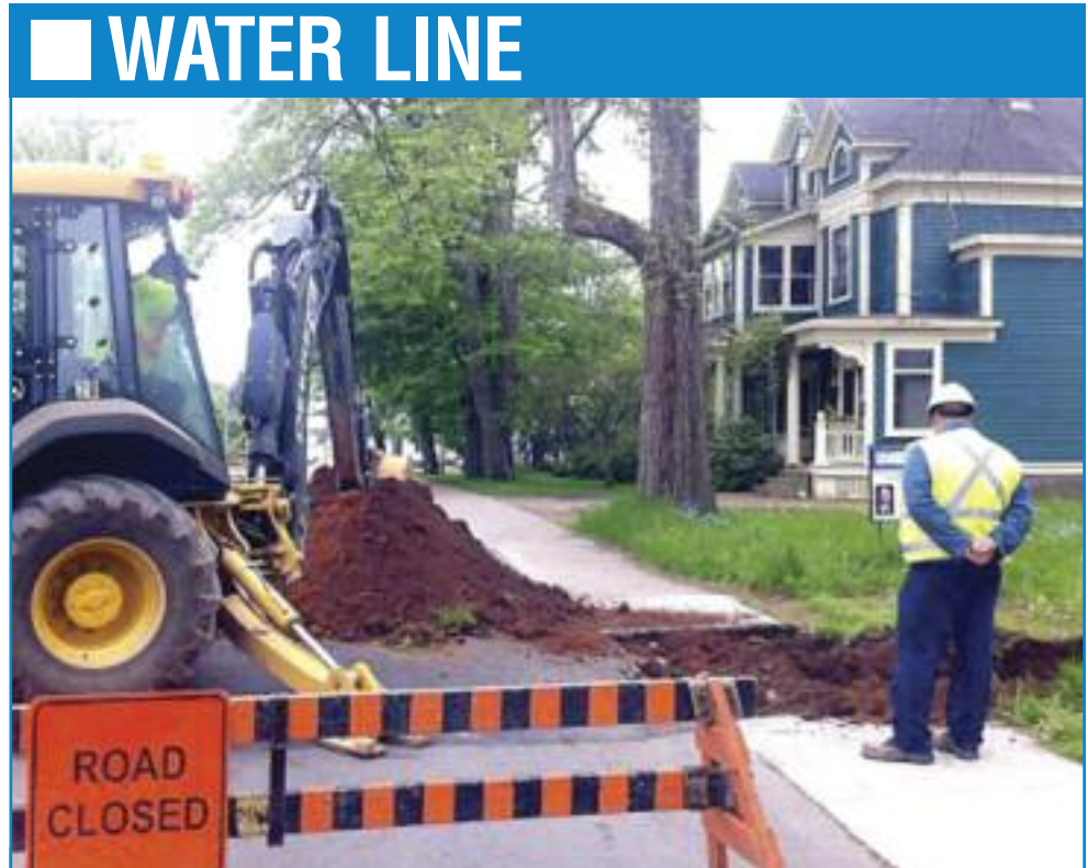
Spring Street in Amherst, Nova Scotia was closed for a bit on the morning of June 2 as crews fixed a water line in front of a vacant home. (Photo: Darrell Cole/ Amherst Daily News)
