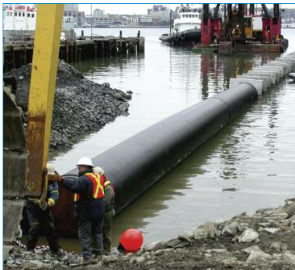
In 2004 a Halifax WTP outfall pipe was floated from Bedford Basin to a location beside Casino Nova Scotia and placed in the water—part of the Halifax Harbour Solutions Project. (Photo: Halifax Water)
