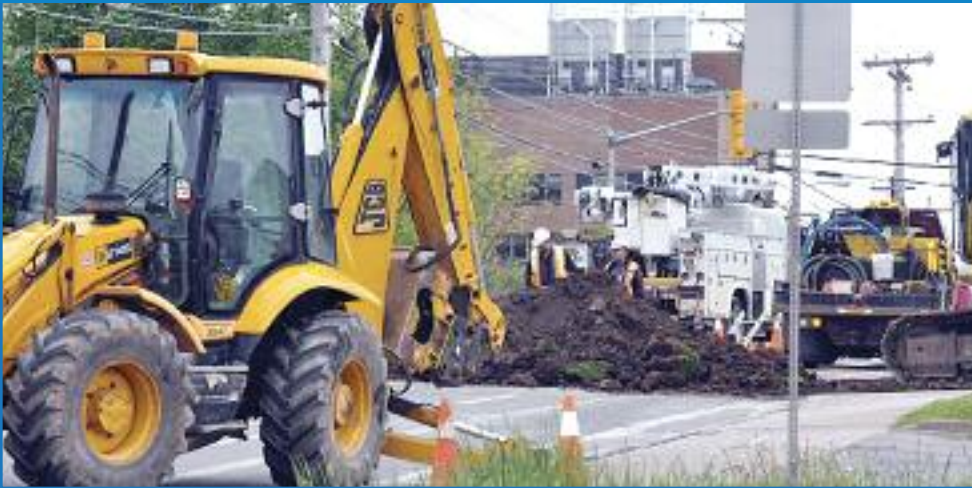
A Town of New Glasgow Public Works crew led by Jeff Grant works on new water valves on the East River Road. (Photo: Jennifer Vardy Little/New Glasgow Daily News)
