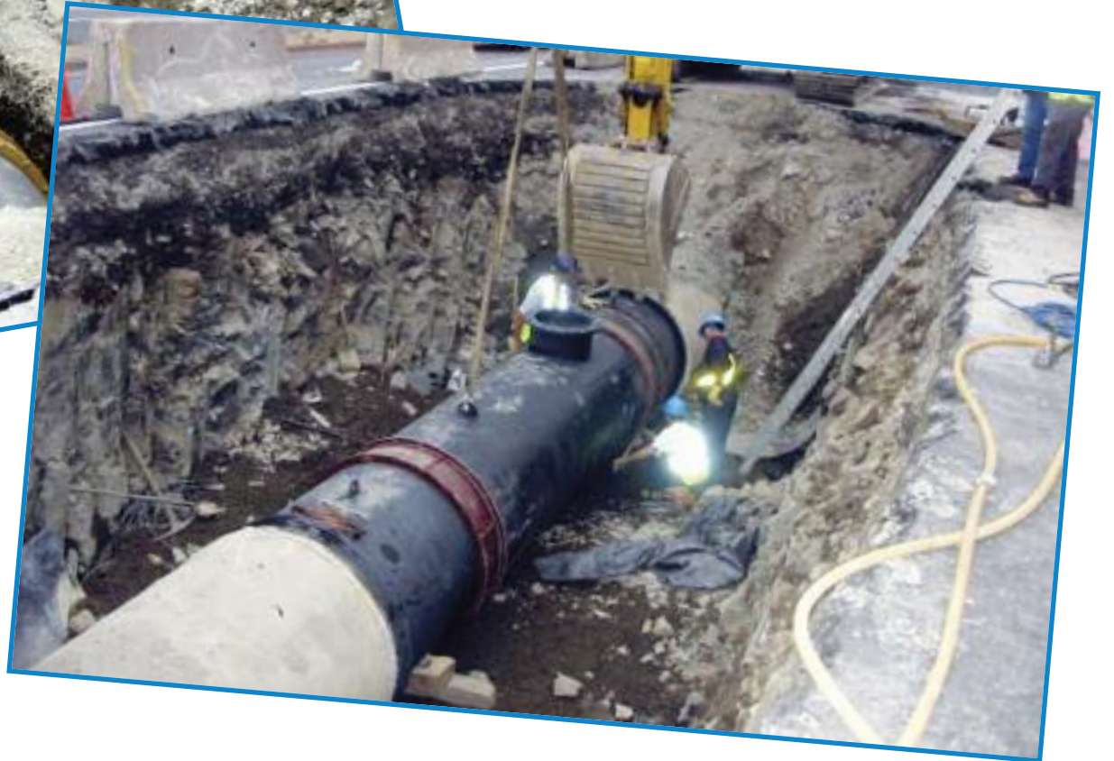
The Dunbrack Street Water Transmission Main Rehabilitation Project for Halifax Water, being conducted by Dexter Construction Ltd., involves sliplining the 1200mm diameter water transmission main with a new 1067mm diameter steel pipe. (Photos: Halifax Water)
