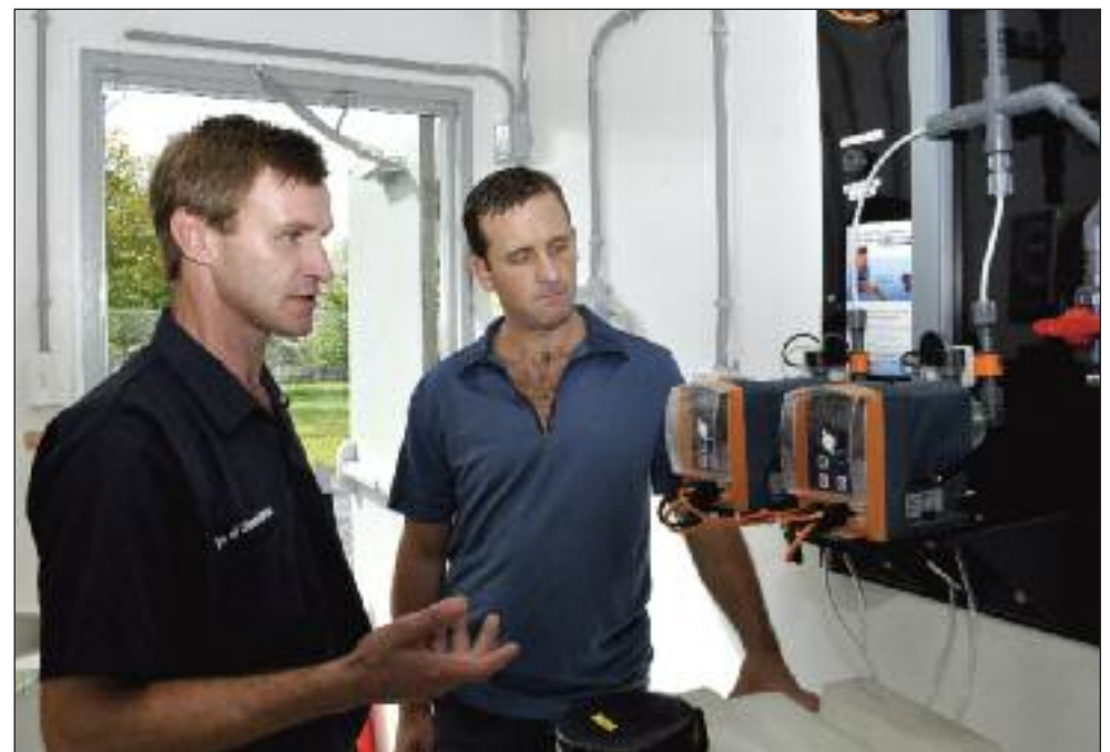
Stewiacke's superintendent of public works Jeff Sibley, left, explains to Mayor Dereck Rhoddy how the new chlorine injector system works at the new water reservoir off of Windcrest Avenue. (Photos: Jason Malloy/Truro Daily News)
