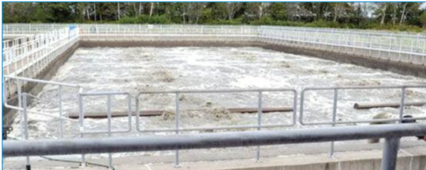
Two Sequence Batch Reactor tanks at Central Colchester Wastewater Treatment Facility in Lower Truro, Nova Scotia are constantly in operation, with each containing 4.5 million litres (one million gallons) of aerated liquid waste. (Photo: Harry Sullivan/Truro Daily News)
