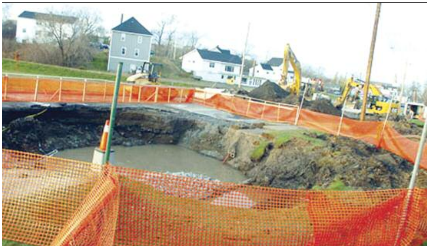
Hosing down the sinkhole. (Photo: Adam MacInnis/ The New Glasgow Daily News)
