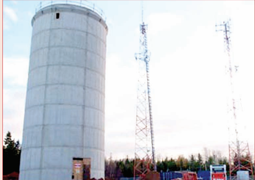
Sackville, New Brunswick's new water tower, which is expected to be completed by early next summer, will provide the town with an additional storage capacity of 550,000 gallons of water, which will offer increased protection in the case of a major fire in the community. (Photo: Sackville Tribune Post)
