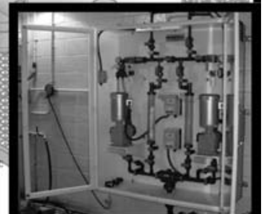
Fredericton Area Pollution Control Duplex Chemical Dosing System with Custom Enclosure
