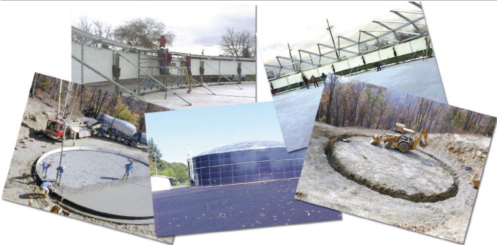
The design, installation and servicing of the new facility is being handled by Greatario Engineered Storage Systems (GESS) of Ontario. These Greatario photos depict the general construction process involved with erecting a reservoir such as the one created in Memramcook.
