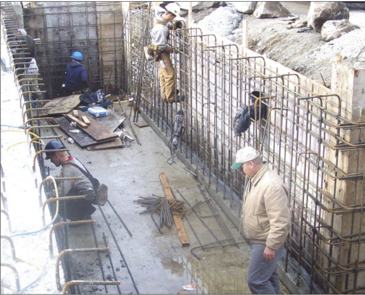
In November, construction on the concrete foundation for the new dissolved air flow flotation (DAF) system was underway.
